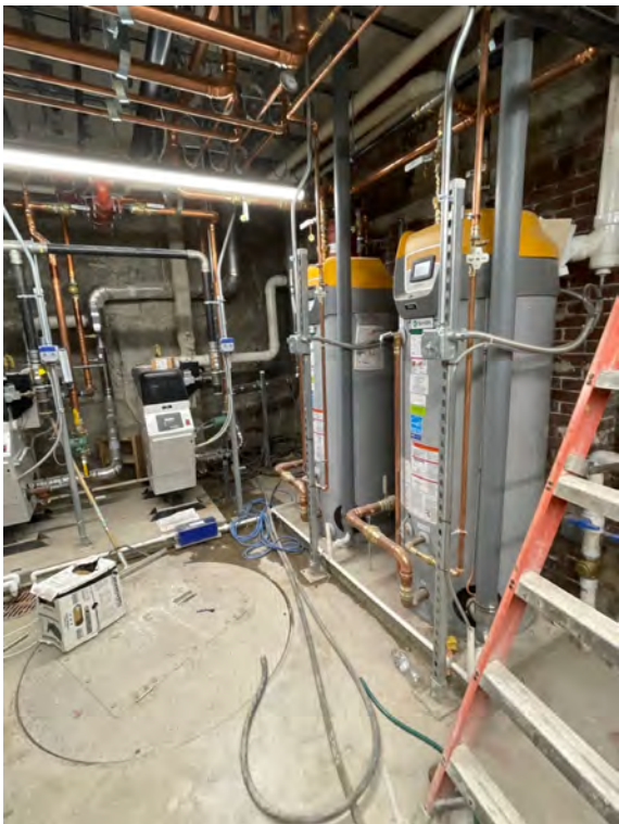
Description: Basement of existing building boiler room, equipment, power
