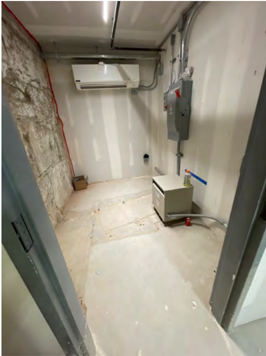
Description: Basement of existing building, elevator, machine room, electrical disconnect, and transformer installed
