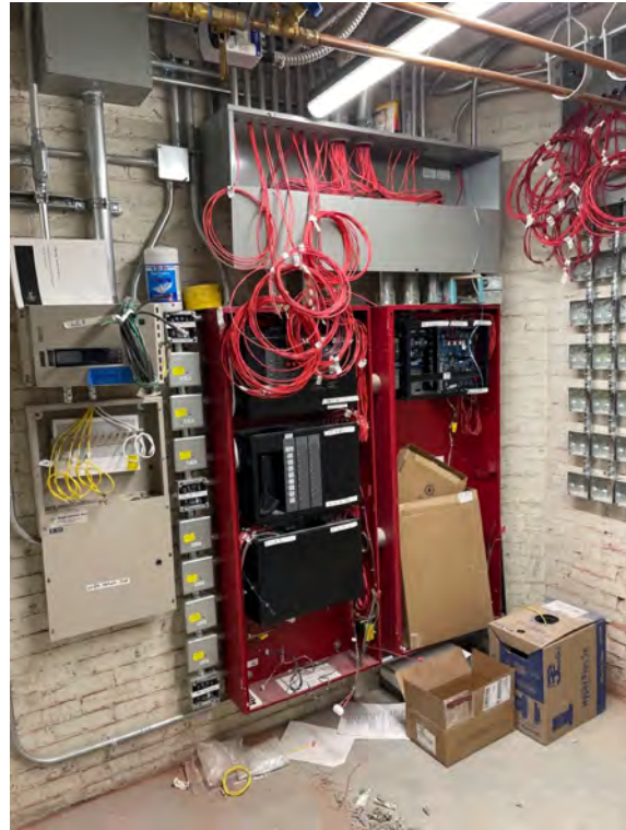
Description: Electrical room fire alarm cabinet
