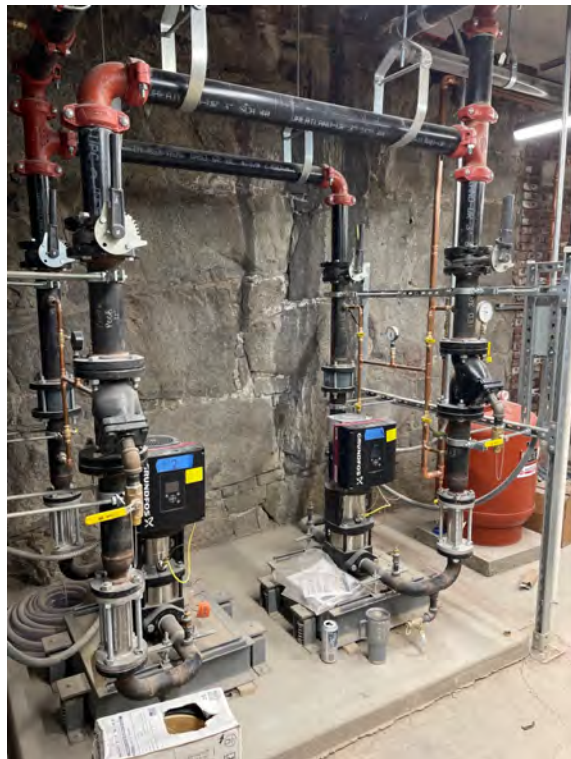
Description: Circulating pumps appear to be operational
