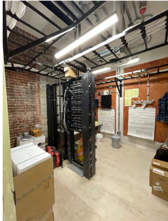
Description: Third-floor existing building, communication wiring, and racks installed
