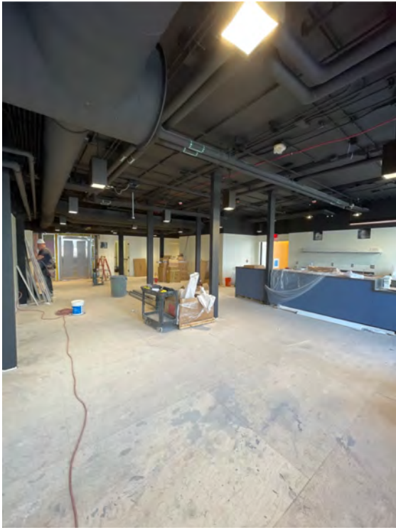
Description: Second floor, existing building walls and ceilings and columns are primed and first coated
