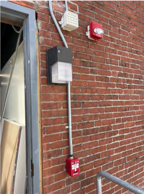
Description: Low roof fire alarm and exterior wall pack
