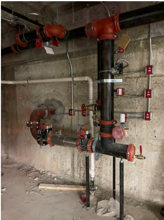
Description: Basement of addition/fire, suppression, main, and valve work
