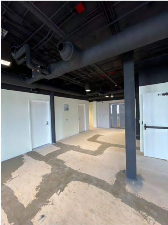
Description: Third floor existing building/wall ceilings and columns, primed, and first coated
