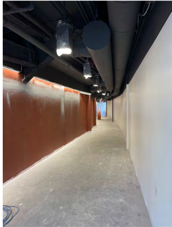
Description: Third floor addition north Corridor walls and ceilings are primed and first coated
