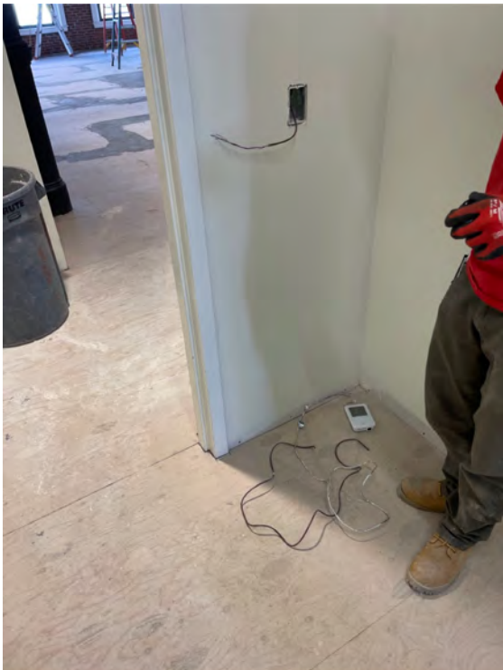
Description: Third floor existing building control wiring in device installation in progress
