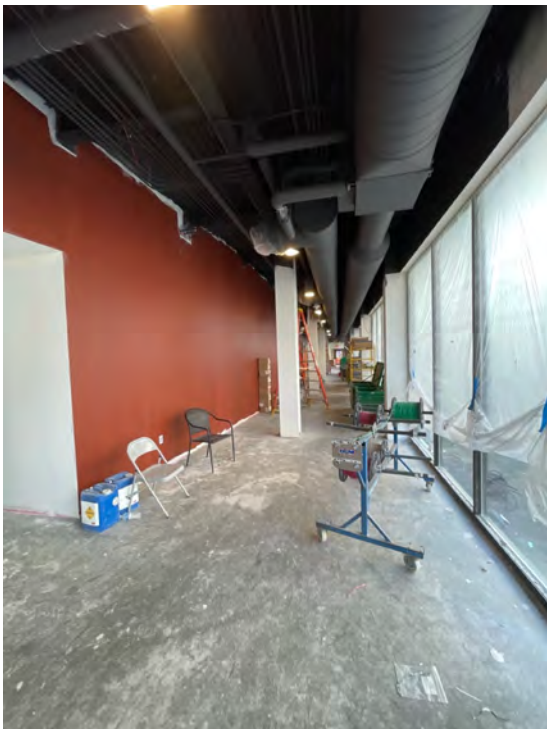
Description: First floor, addition, North Corridor sheet rock appears complete/walls and ceilings are primed and first coated
