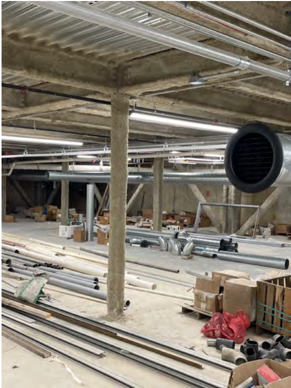
Description: Basement of addition/registers grills, and diffusers
