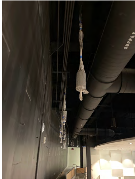
Description: Fourth floor, addition north elevation walls and ceilings are primed and first coated light fixtures installed
