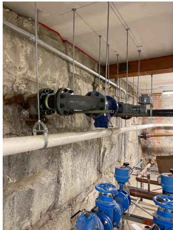
Description: Basement of existing building fire, suppression service/final connections, appear complete
