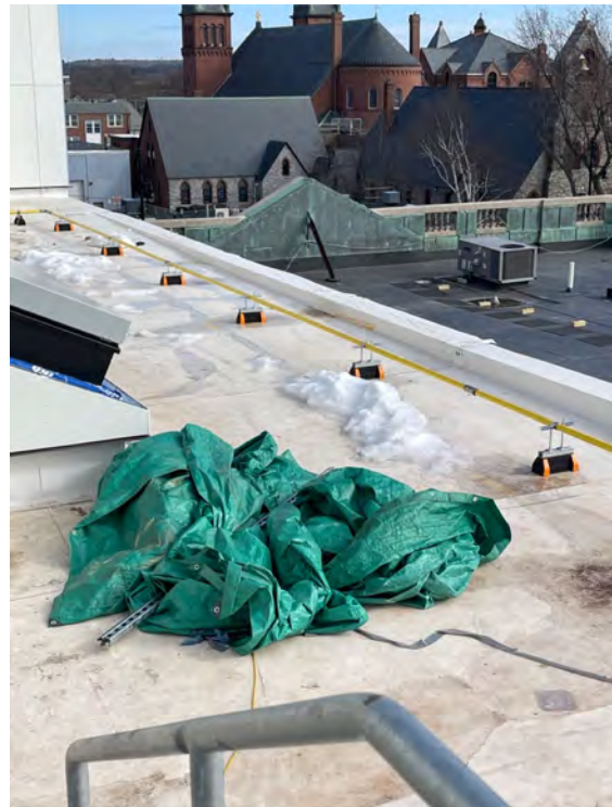
Description: Low roof gas piping
