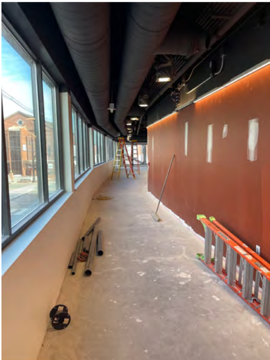
Description: Second floor, addition North Corridor/walls and ceilings are primed and first coated
