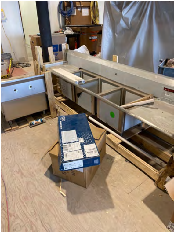
Description: First floor existing building stainless steel plumbing fixtures
