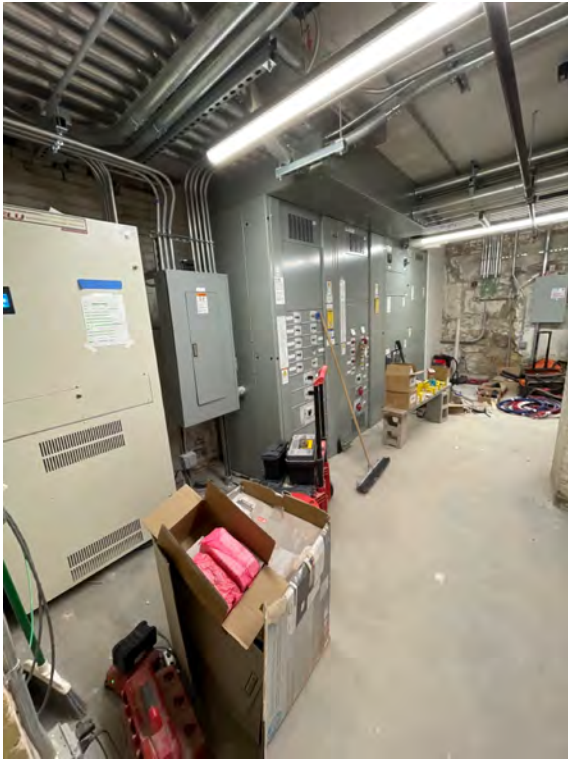
Description: Electrical room
